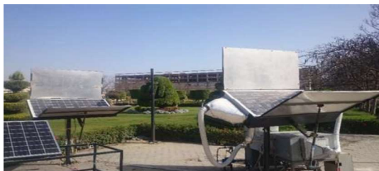
Fig 13 Two Monocrystalline photovoltaic modules with different cooling
